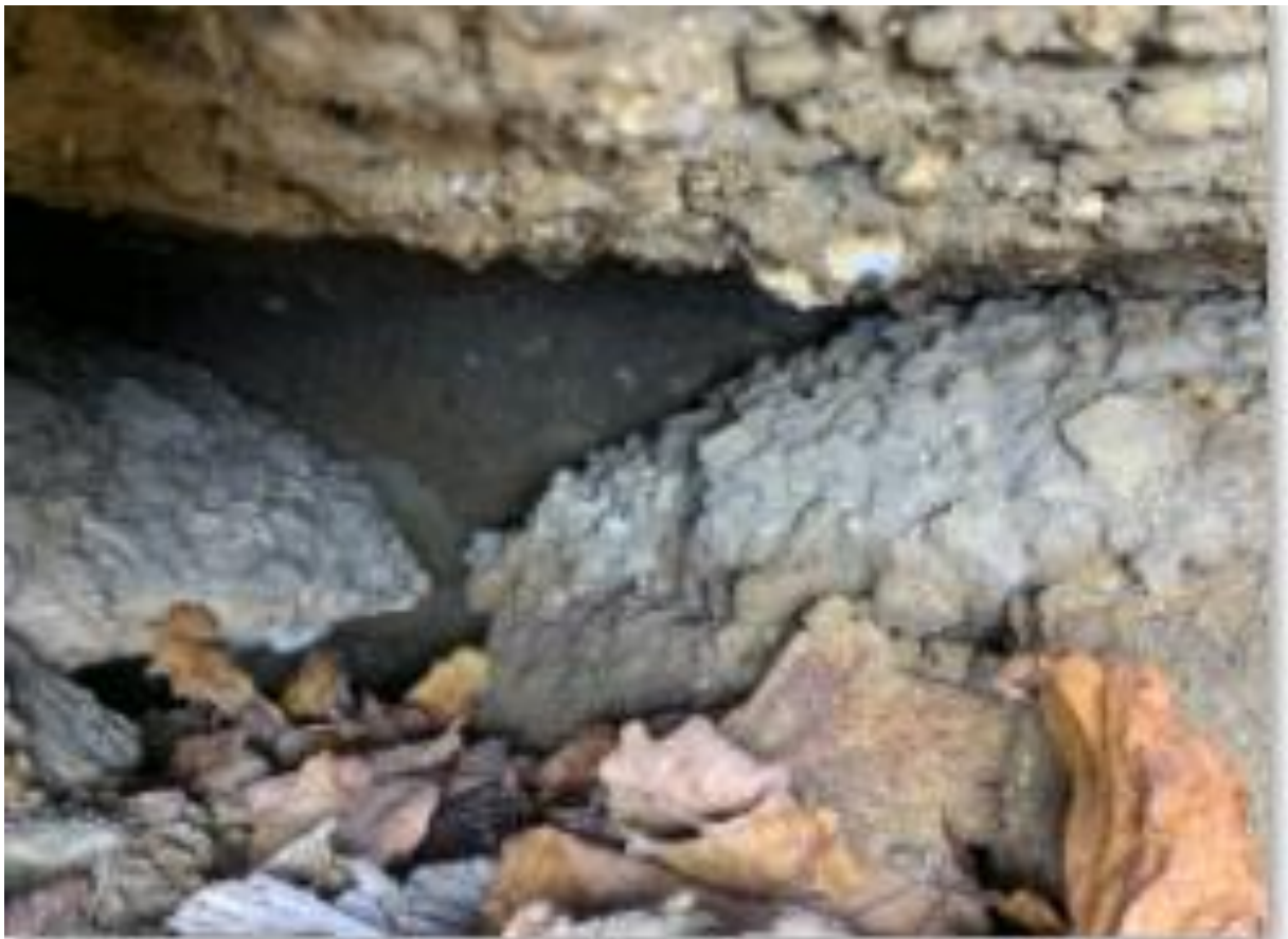
Photo 9: Site visit photos – location of paviers removed to investigate substrate. Back of pool tank visible
